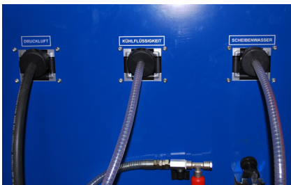
Built in hose reels
