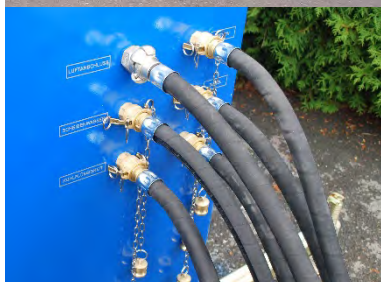
Preinstalled quick-couplings for tank line
